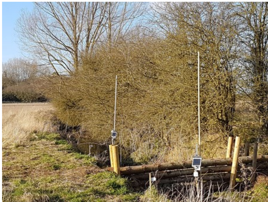
Figure 17 Leaky dam at Spains hall estate on Blackwater river with upstream and downstream water level sensors
